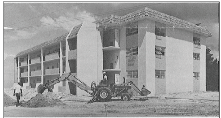
Recent photo shows that our Phase I buildings are structurally complete and getting ready for first occupancy to begin in September.
